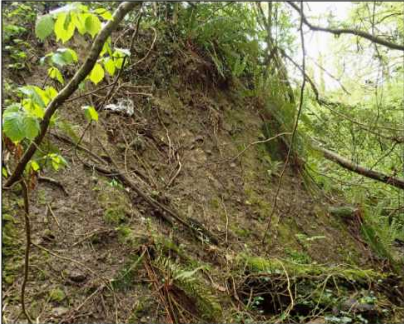
Plate 2. A substantial recent stream bank collapse in Coneyburrow Wood.
