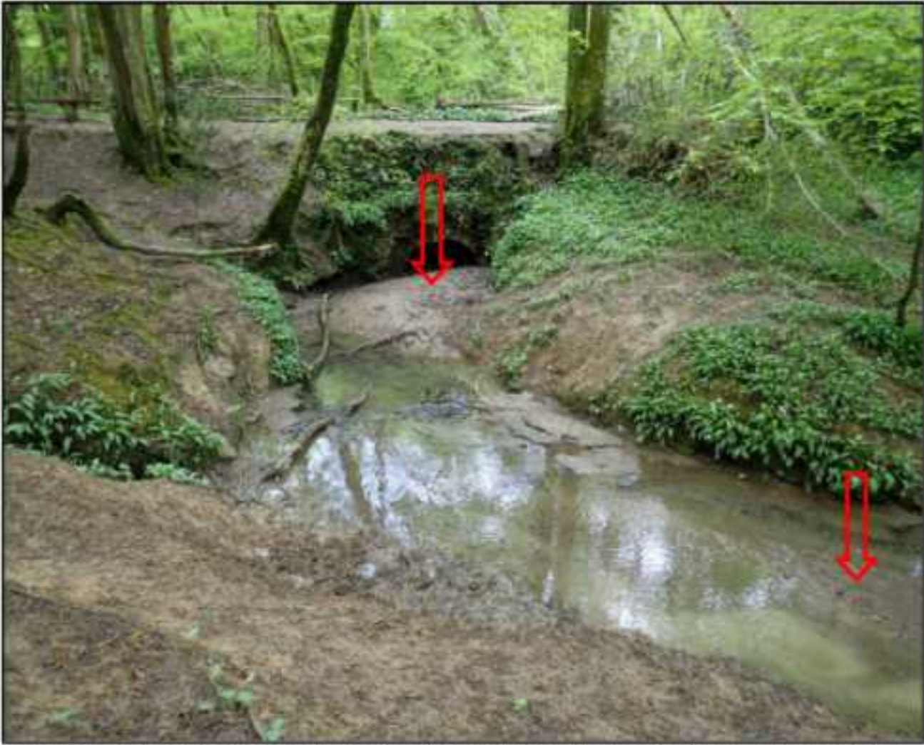
Plate 3. Banks severely eroded by dogs/people near the footbridge in Marline Wood. Prominent silt bars are also present above (arrowed) and below the bridge
