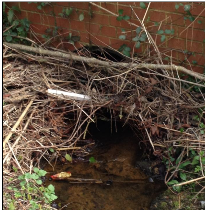
Figure 6 – Photo of debris build up against culvert
