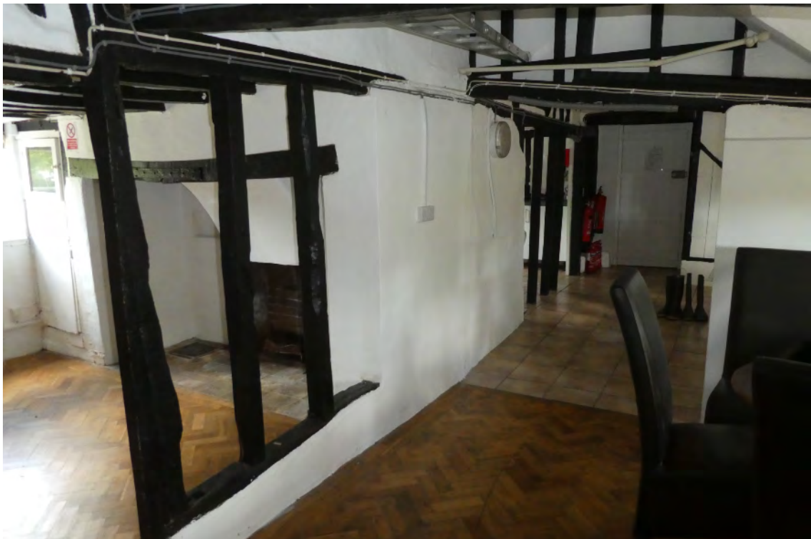
6. Interior of rear leanto looking east showing rear wall of phase 1 main frame, west end post left and intruded phase 2 chimney centre.
