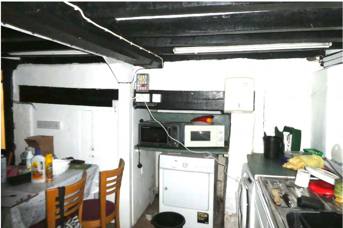
14. Phase 2 east cottage kitchen (service room in phase 1 building) looking west showing inserted phase 2 inglenook fireplace, phase 1 girder ceiling top.
