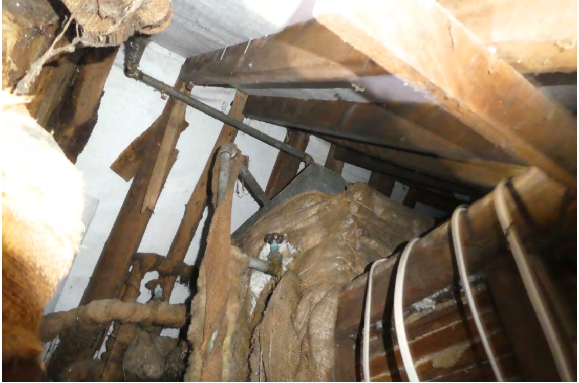
13. Phase 1 roof looking east showing paired rafter construction (lacking a ridge board), inserted chimney left, later inserted partition adjoining a lowered ceiling bottom right.
