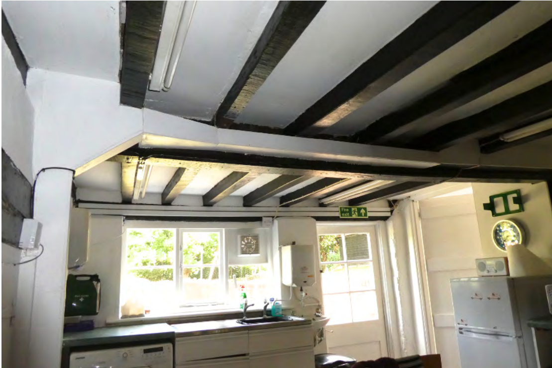
5. Phase 1 services room (present kitchen) looking north showing first floor central girder construction.
