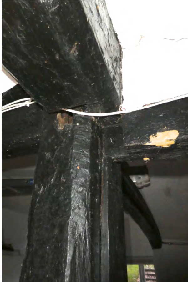
7. Phase 1 west end rear post from inside phase 1 kitchen showing mortise for removed cross beam beneath phase 2 inserted lapped cross beam. Leanto beyond.
