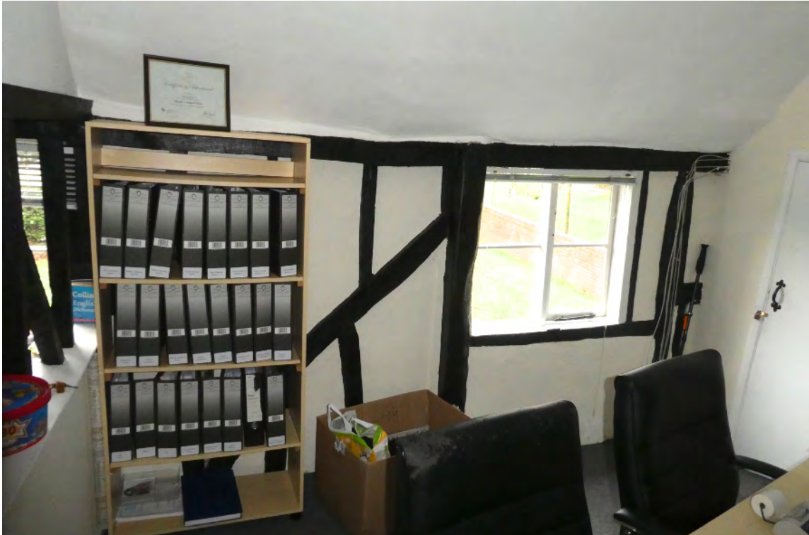
10. Inside of front wall showing front west post of phase 1 main frame centre with phase 1 small square panel right and raised cill for former window beyond stud. Phase 2 stud and raking strut construction left.
