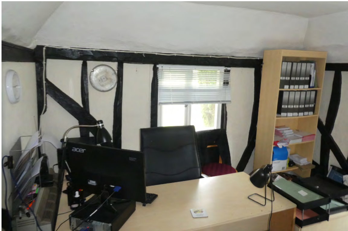
18. Phase 2 added west bay looking west in first floor chamber showing raking strut and stud construction and bowl shaped jowl to head of principal post left.
