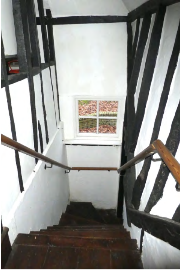
19. Phase 3 stairs looking to rear, main part of phase 3 extension left, return leanto right.
