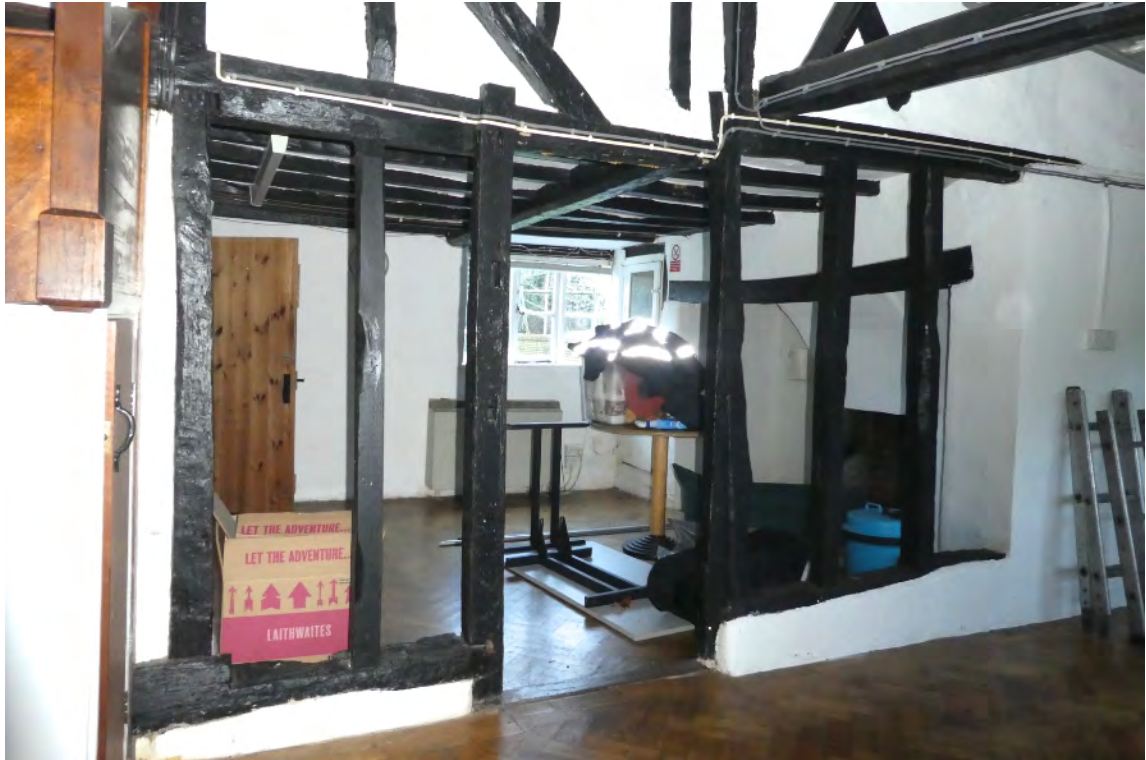
15. Rear leanto looking north east towards front showing phase 2 west cottage kitchen and inserted inglenook fireplace. Phase 2 replacement first floor construction over.
