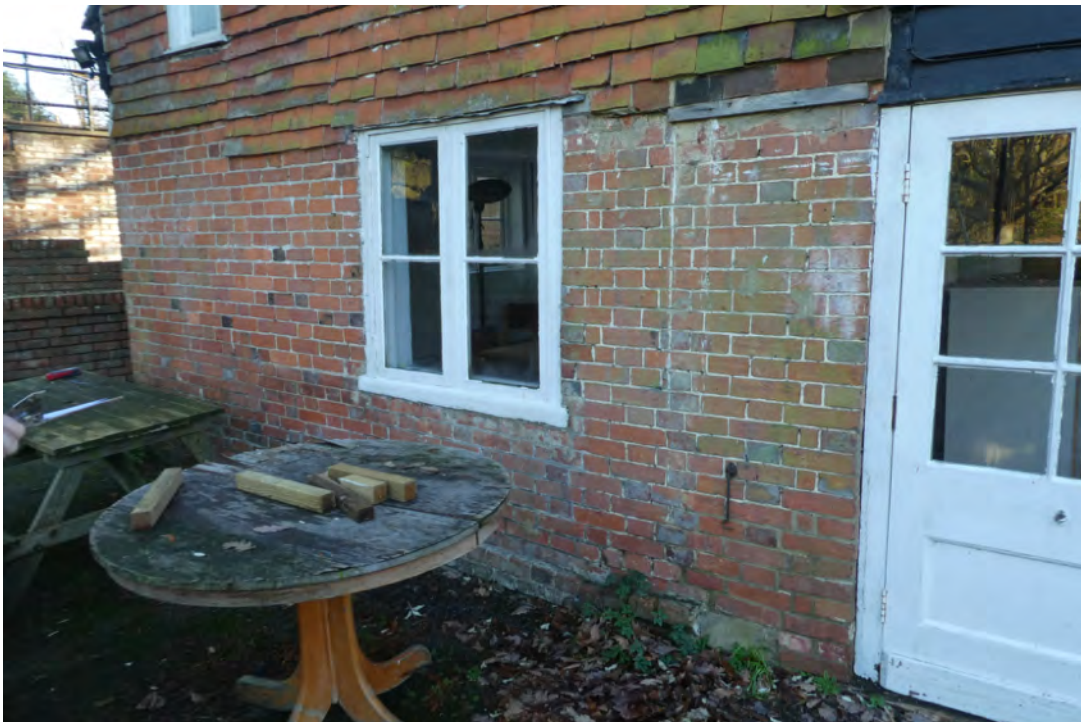
2. Detail of area at front elevation no longer proposed to be enclosed by a link structure to the proposed new building.
